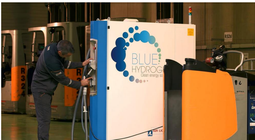
Figure 2: Demonstration of the principle of the hydrogen charging station with a dispenser installed onsite
