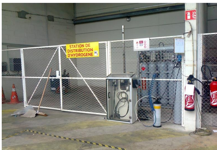
Figure 7: Air Liquide transfilling system
